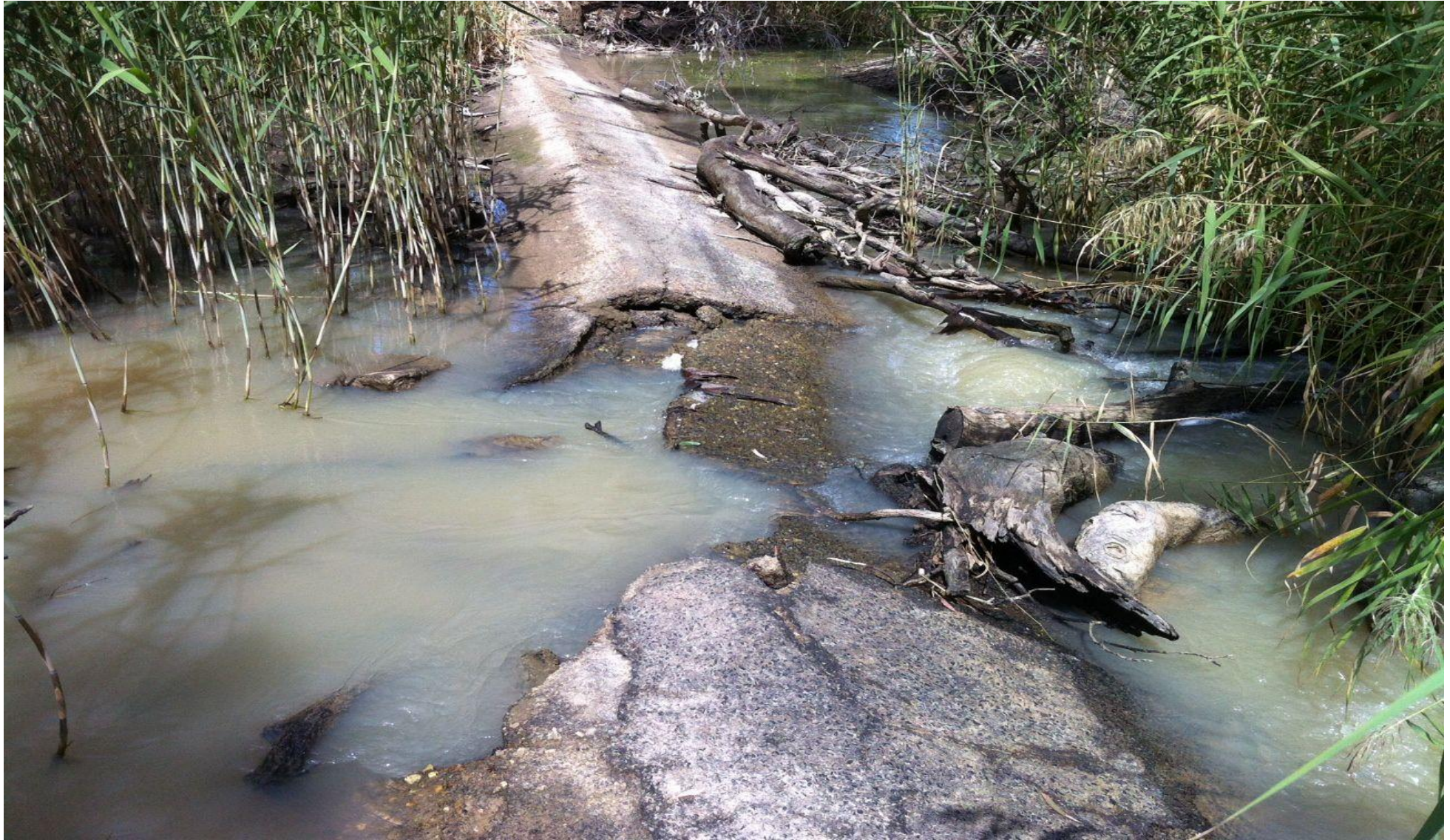
Wimmera River – Damaged Sill
