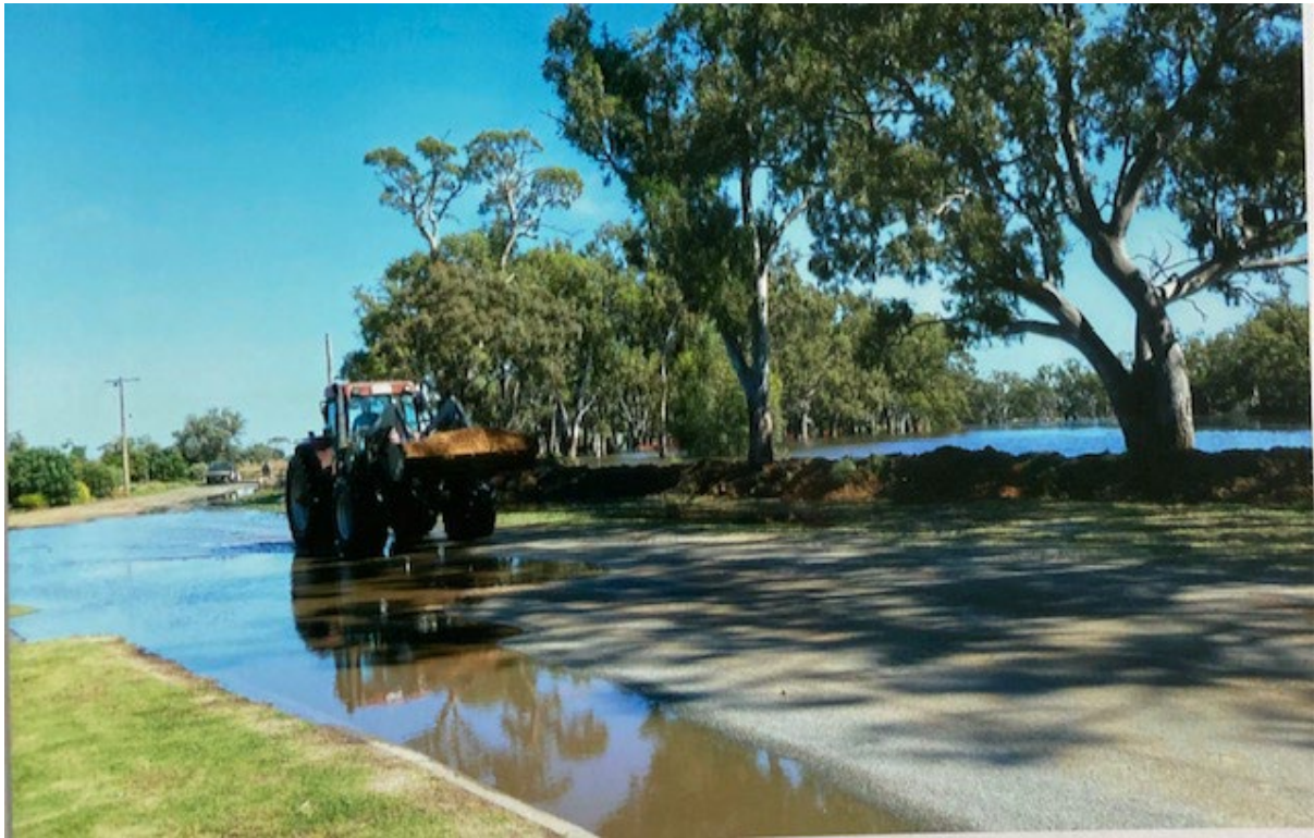
Photo 8 - 18/01/20011 Levee banks being constructed along the Yarriambiack Creek, failing to manage inundation
