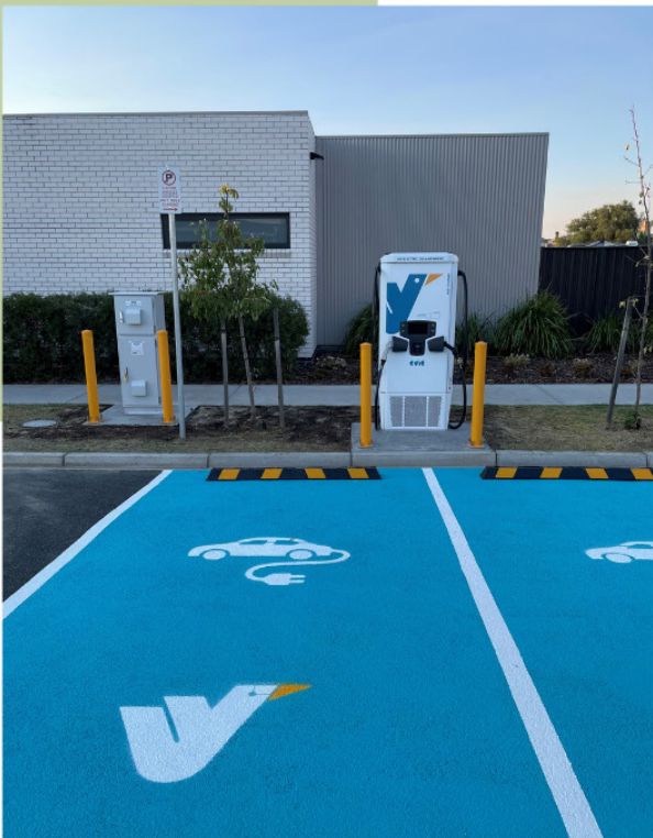
EV Charging Station
